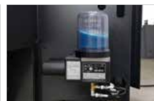
Lubricating Oil Tank
